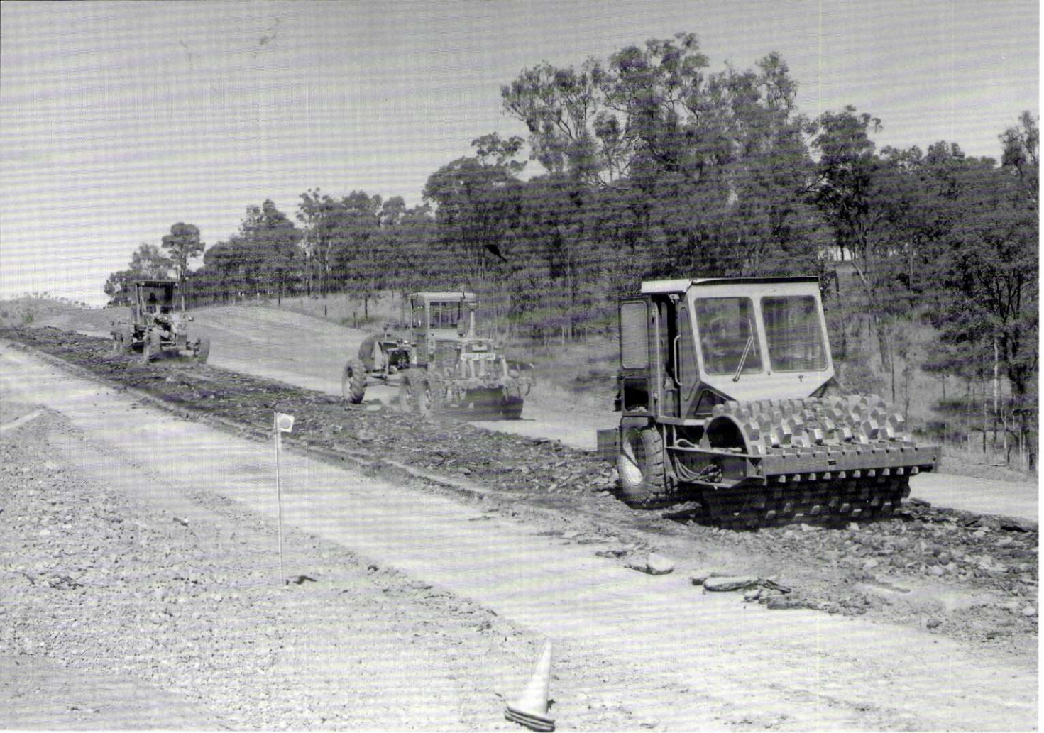
Road construction work on the Brisbane Valley Highway near Ottaba south of Toogoolawah. 1987.
