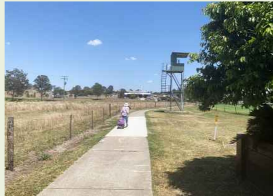
Shared path - used by wider community - isolated damage to be repaired
