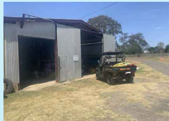
Race Club Maintenance Storage Shed - poorly located and insufficient size to accommodate all infrastructure
