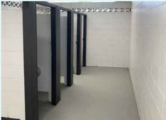
Amenities building (internal female cubicles) - require upgrade
