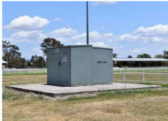
Padmount transformer - suitably sized to service site
