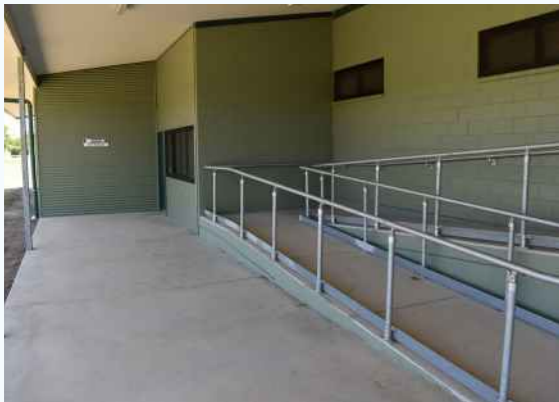
Ken & Mary Nunn Pavilion (Toilets and Showers) - newly constructed and fit for purpose
