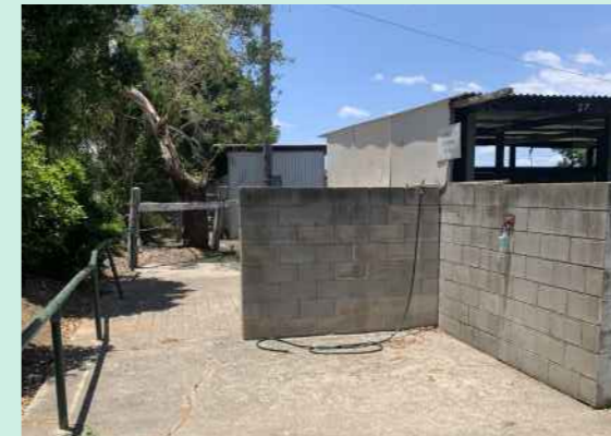
Wash Bays - insufficient number and worn concrete, requires upgrade and additional
