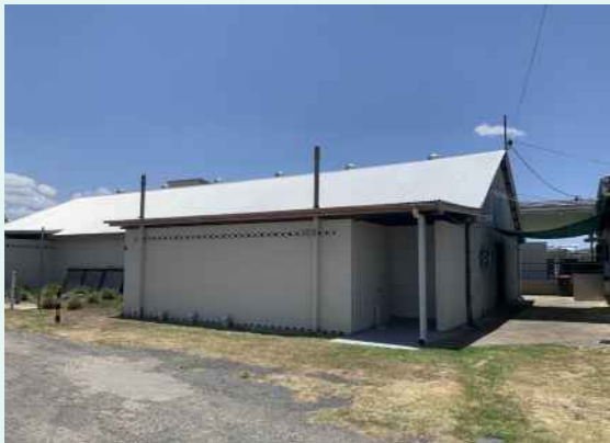
Amenities building - Aging and requires upgrade
