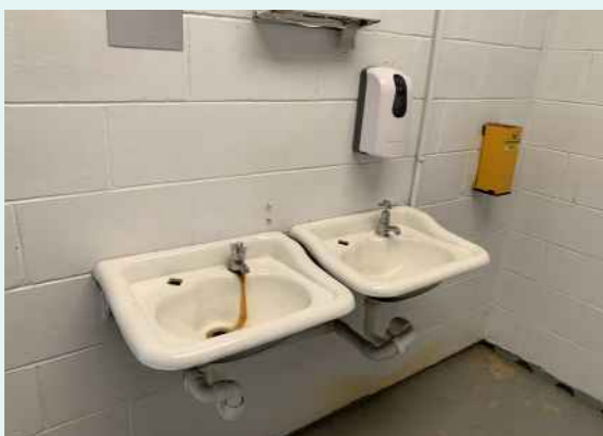
Amenities building (female) - requires upgrade
