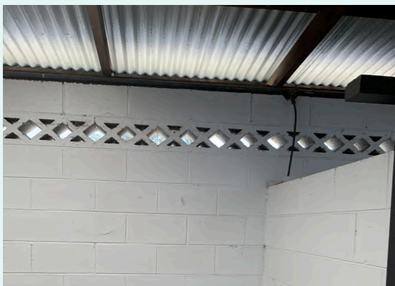
Amenities building - basic construction materials - Aging and requires upgrade
