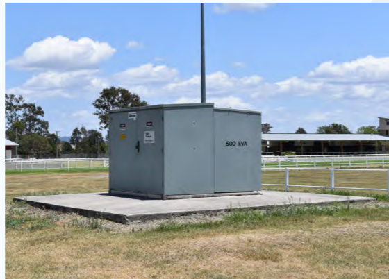
Padmount transformer - suitably sized to service site
