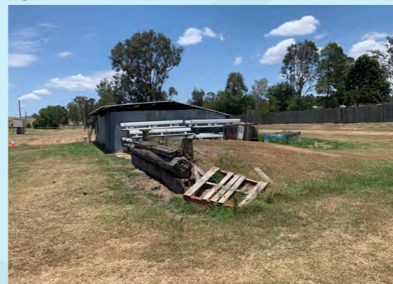
Loading Ramp and Pony Club Storage Shed - no longer required in this location and not fit for purpose
