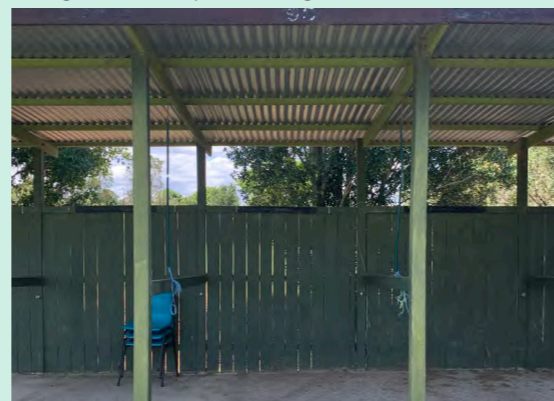
Tie Up Stalls - aging and requires renewal
