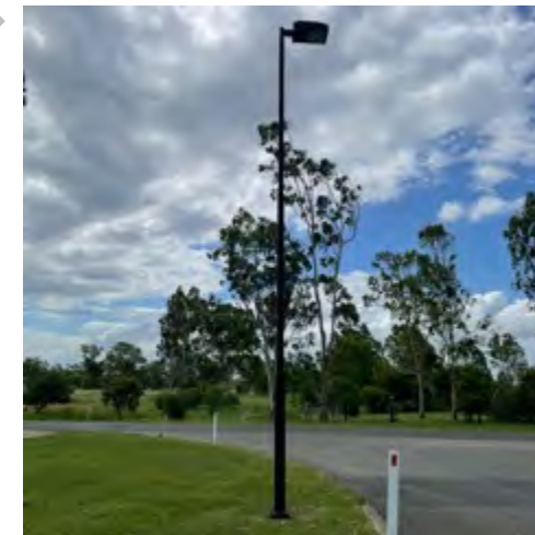
Entrance Lighting Light posts featured throughout entrance leading to car park
