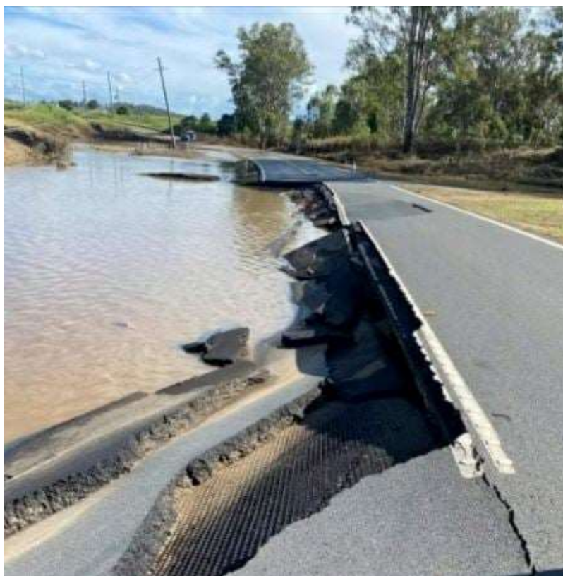
Figure 6: Damage on the Brisbane Valley Highway south of Geoff Fisher Bridge from the Feb-Mar 2022 Severe Weather
