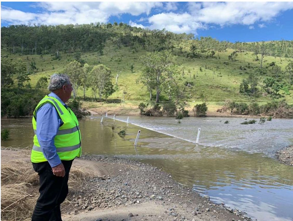
Chair of the LDMG inspecting damage post the Feb-March 2022 Severe Weather Event (March 2022)
