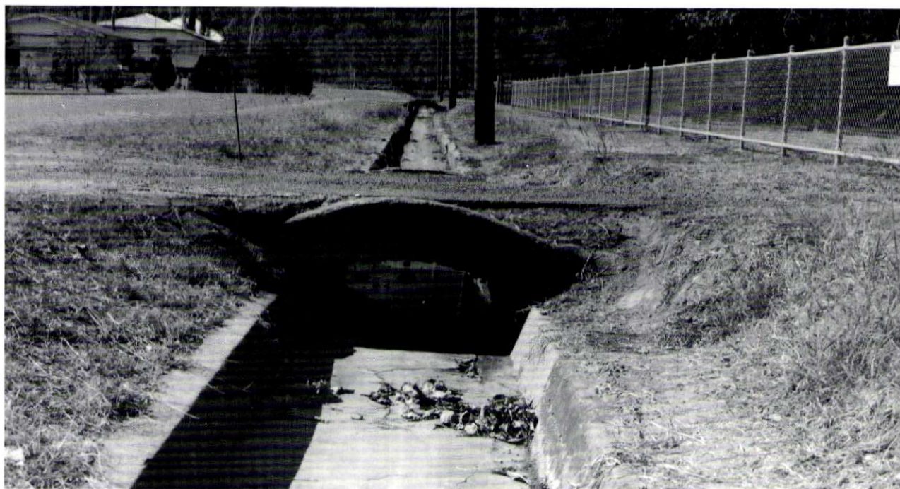
Substantial concrete drain dug in 1932 down Highland Street and past the post office down to the creek to alleviate part of Esk's drainage problems. (1987.)
